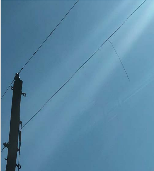
^ Owen County (Frayed copper weld wire)
